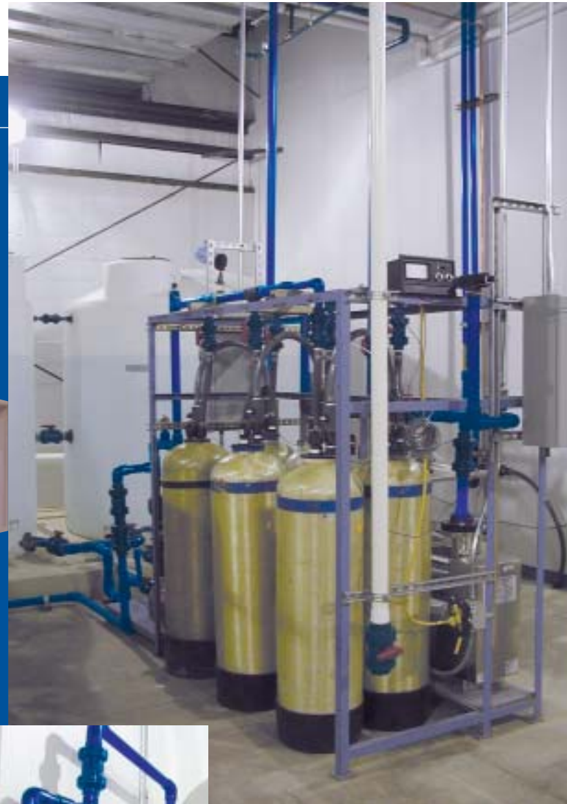
Pretreated water is sent through a reverse osmosis system with a design flow rate of 20 GPM prior to deionization.
